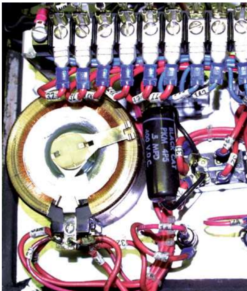
Fig. 2 shows the variable transformer from the inside of the control panel.
